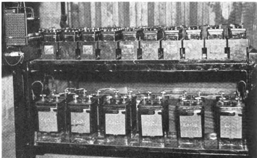
The 115-volt C. T. C. line battery and the local battery in the office at Aurora
