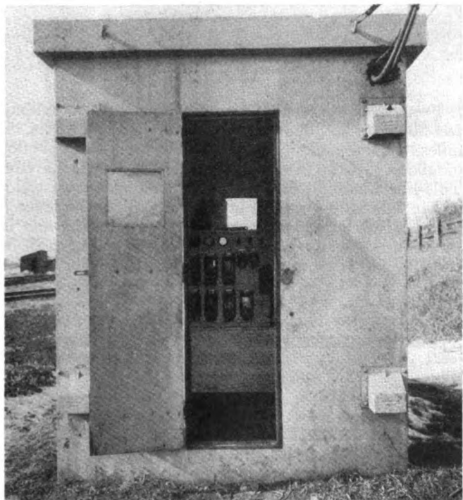
The relay, batteries, etc., are located in small concrete houses
