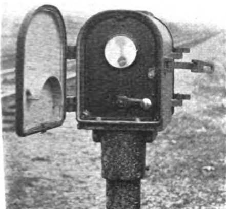
Electric lock with door open
