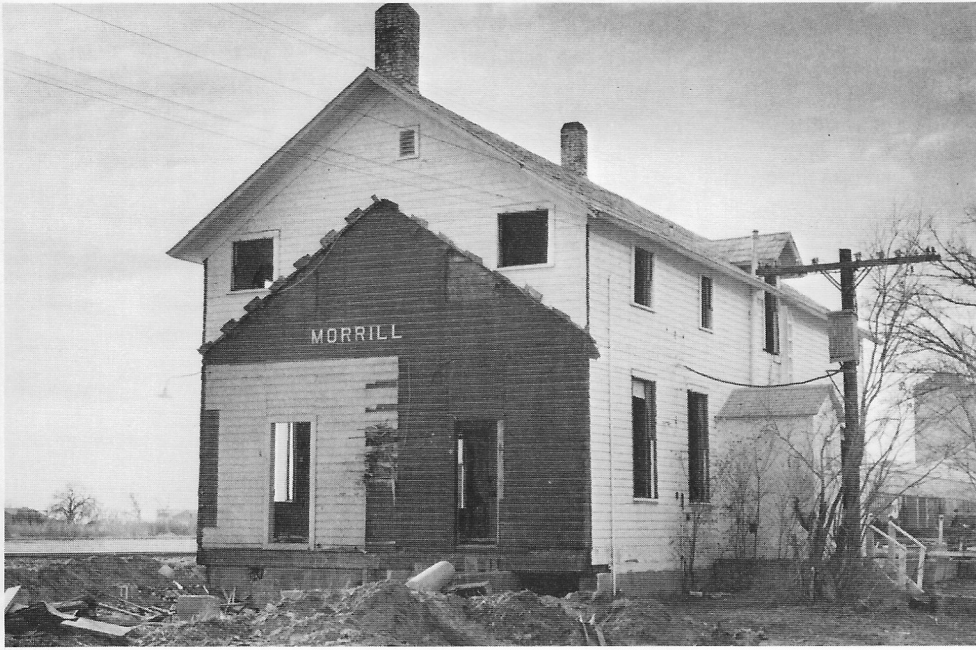
The final fate of the Morrill BN depot was similar to many other frame depots across the Midlands that were dismantled so that building materials could be salvaged. By November 1981, dismantling of the Morrill building had progressed to where the one-story freight room had been removed. The painted-on station name that was exposed by this action indicates that the freight room had been added later to the original two-story portion. — Scottsbluff Star-Herald
